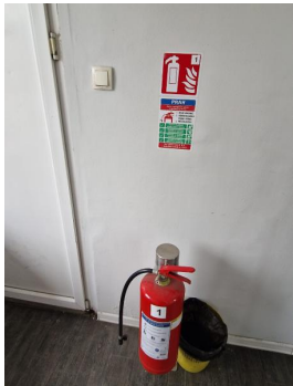
Fire safety at site 2.jpg
