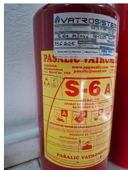
Regularly checked fire extinguisher.jpg
