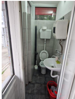
Toilets for the security at site 2.jpg
